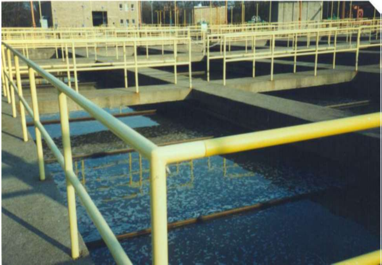
Fig17 primary settling basin
