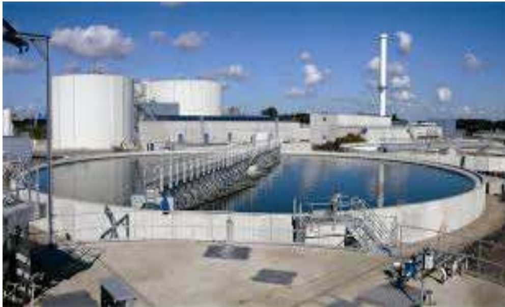
Fig 19 waste water treatment plant
